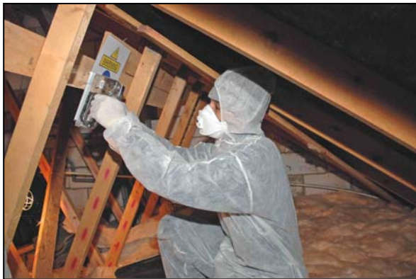
Working Herts personnel insulating a loft—social enterprises offer a high quality service
